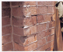
清水磚砌的灰泥凸縫細部。 Protruding seams made of plaster between layers of bricks in detail
